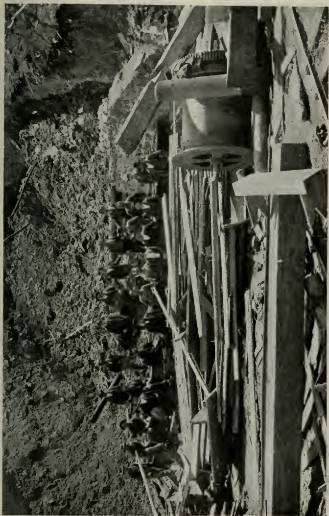
Wreck of Power House at Opening to No. Four Mine.
